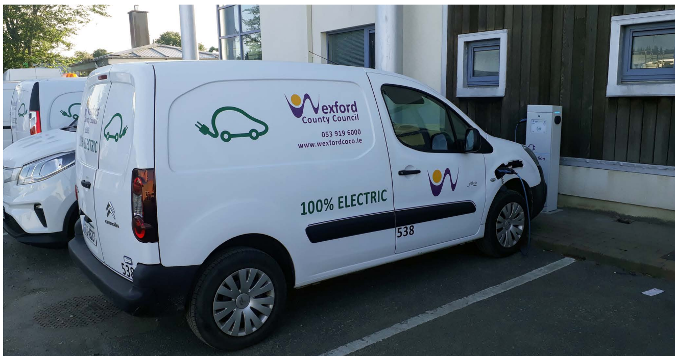
Figure 11: Wexford County Council – 7kW Single phase EVCP installed in a machinery yard (Source: Wexford CC)
