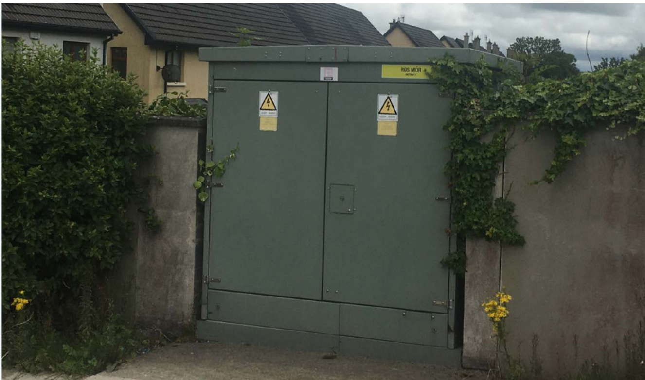
Figure 25: Typical Unit substation in a housing estate (Source: ESB Networks)
