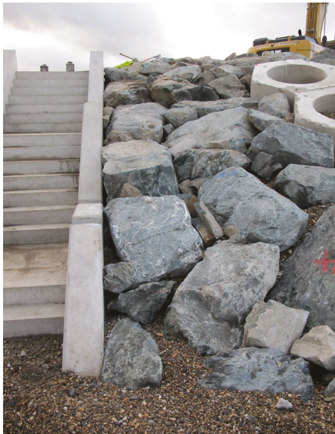
Figure 9 Seabee revetment works at termination of hard defences at the Murrough and new beach access concrete steps
