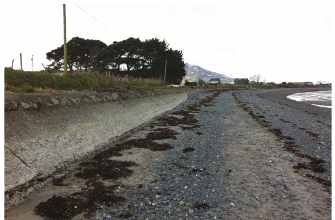
Scour at the toe of revetment at Greenore Co. Louth (Arup)
