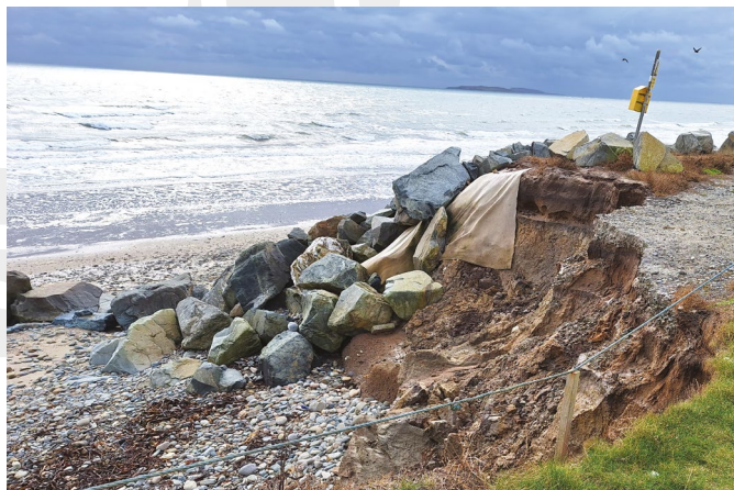
Erosion of access road following storm event, Seaview, Co. Wexford (CARO)
