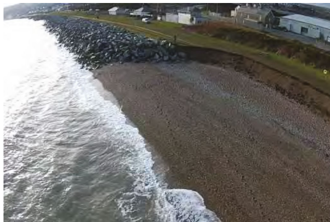
Erosion of coast adjoining revetment, The Murrrough, Co. Wicklow (Wicklow County Council)
