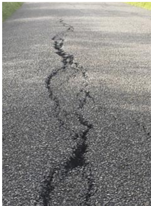
Figure 5.21: Road cracking following drought in 2018.
