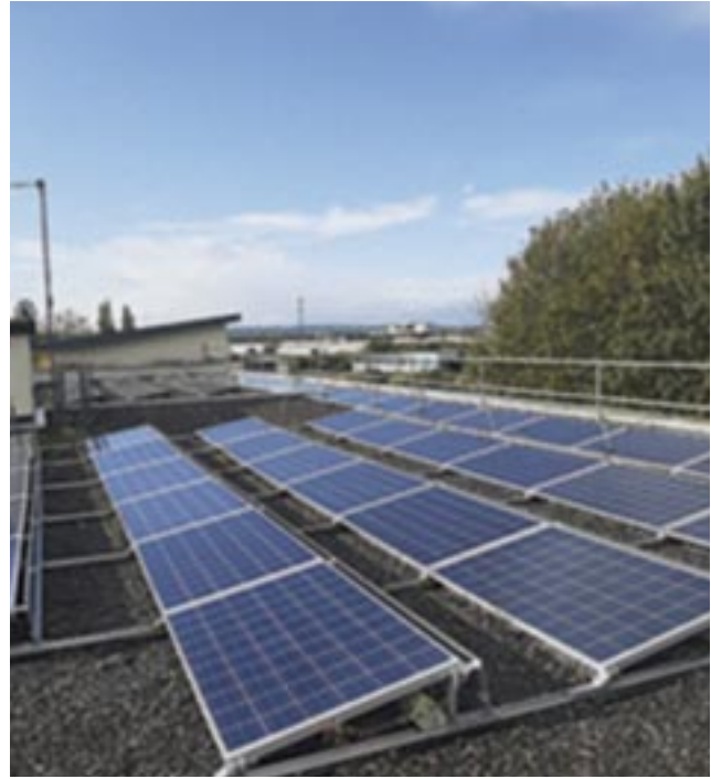
Figure 5.14: Solar panels on Carlow County Hall.
