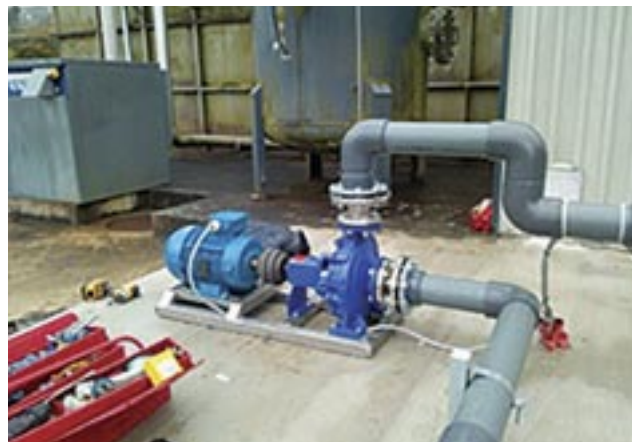
Figure 5.18: Blackstairs GWS hydropower technology.
