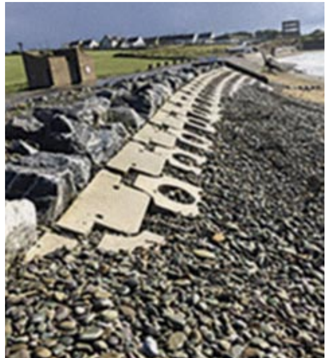
Figure 5.37: Erosion control armour block – Garrettstown Beach, Co. Cork.
