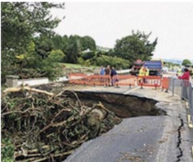
Figure 5.27: Road damages – flooding, Inishowen, 2017.
