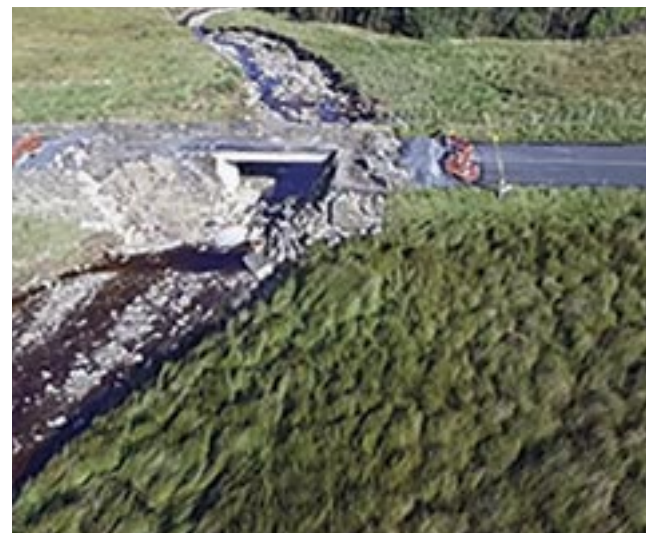
Figure 5.28: Aerial view damages – flooding, Inishowen, 2017.
