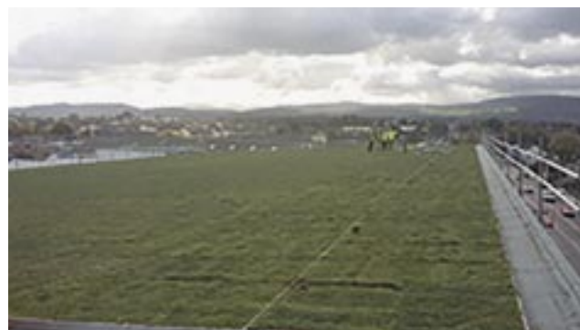
Figure 5.45: Green roof – Dún Laoghaire Rathdown County Council.
