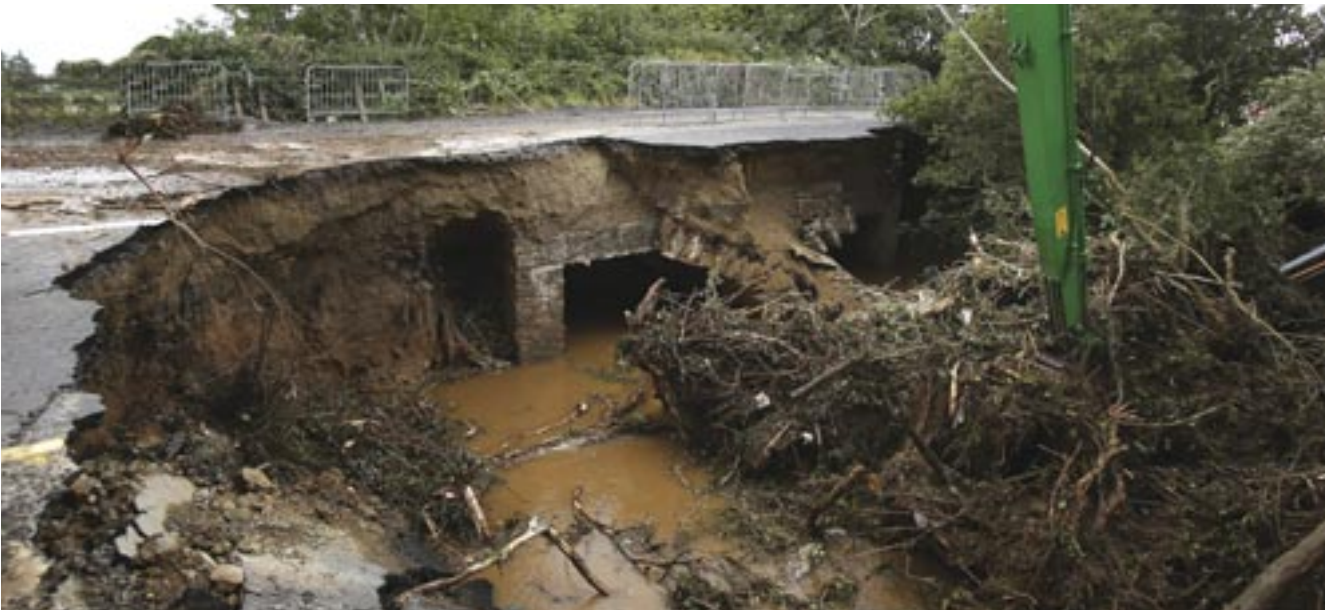
Figure 5.26: Flood damages, Inishowen, 2017.
