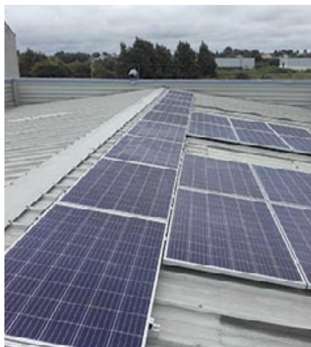
Figure 5.13: Solar PV panels on Roscommon Town Fire Station.
