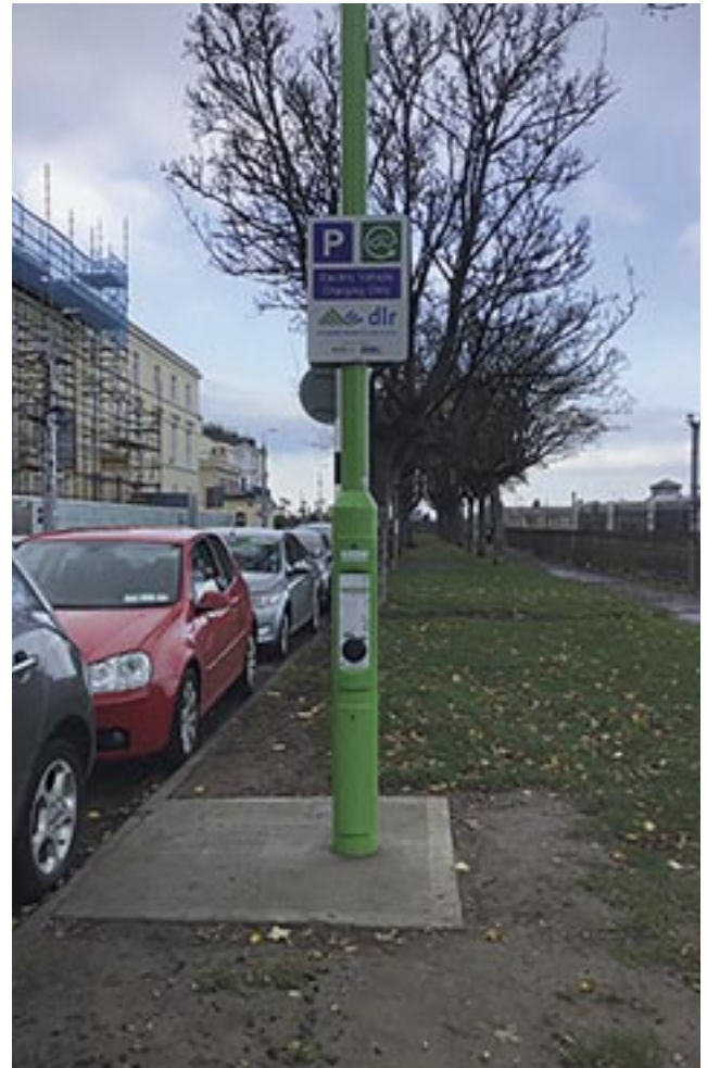
Figure 5.19: EV public lighting charging point.
